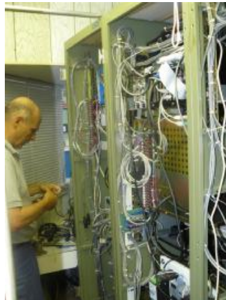
Dave Olson in Control Room
